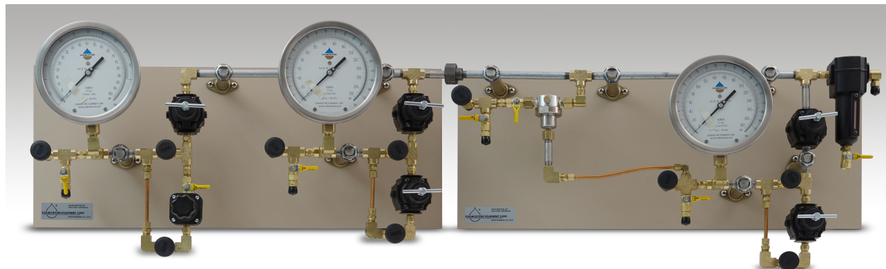
Figure 01 - Typical 0700CG1F123F1 Manifold Setup
