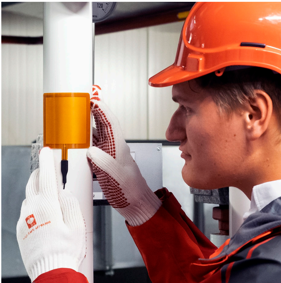
Figure 4.1.1 Example of model FHF05-85X85 foil heat flux sensor being installed for measurement on an industrial pipe. The sensor is mounted on a well-prepared curved surface.
